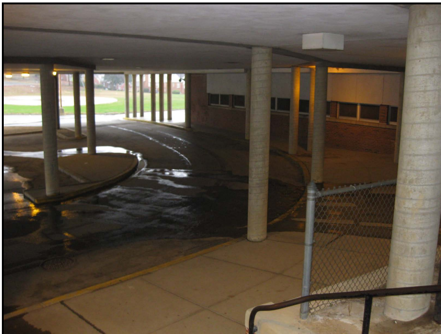
Photo: Fairmont Heights High School, sheltered access beneath northeast corner of school, looking northeast. (December 2009).
